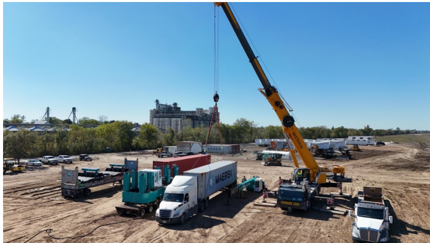
Figure 1 - Ongoing construction of BaRupOn LLC. 701-acre Liberty American Multi-Sourced Power ("LAMP") and Innovation Hub in Liberty Texas, USA.
